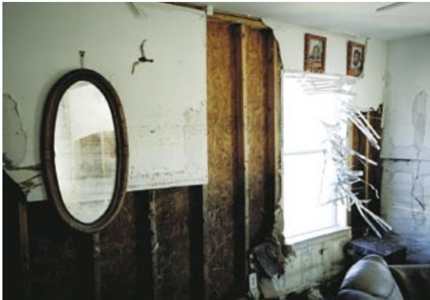
KATRINA STRIPPED the walls to the studs and smashed the window blinds on the first floor of a year-old home in the New Desire development. A mirror that survived reflects further damage.
